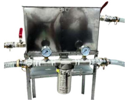
Pilot Filtration Skid
